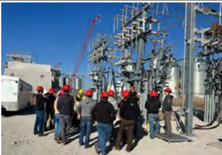
Pictured left: NECC Utility Line students tour a new substation. Our partnership with NECC helps us with employing great staff, which in turn helps us with our mission to have reliable service.
