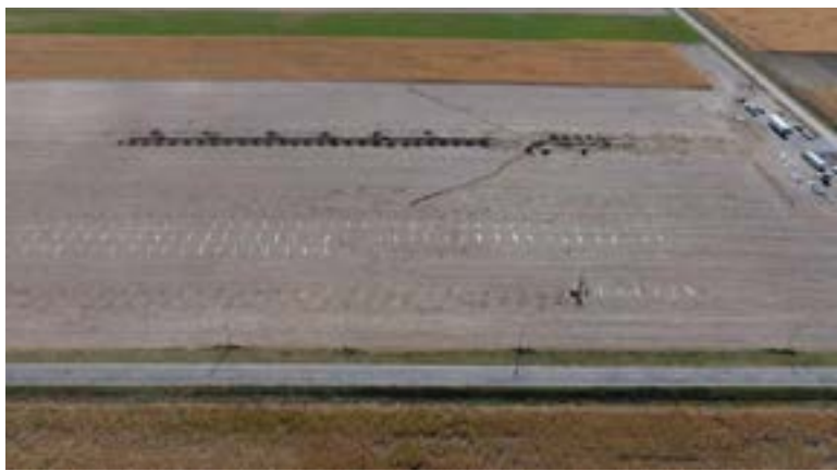
The picture to the left shows an aerial shot of the start of the 3 MW project that is south and west of Norfolk.
