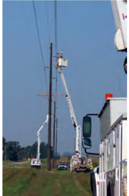
Crews tie in the sub-transmission line for Norfolk Crush - one of 2023 highlights.
