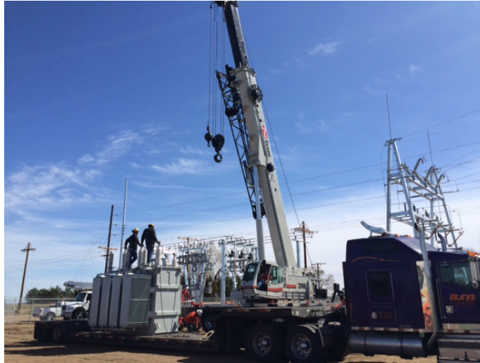
Preparing to set the transformer in the Trease Substation, located 2 miles south and 3 miles east of Orchard.
