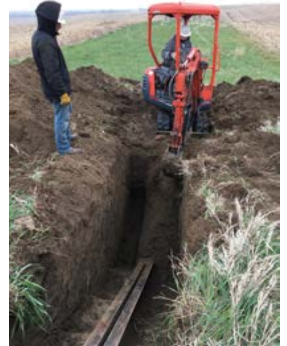
Pictured above: Needmore Tower Service exposed the anchors at ERPPD's communication tower to inspect the integrity of the shafts. The anchor shafts are 20' long imbedded in concrete blocks that are 8-feet deep and are 2' x 2' x 11' long. (Picture credit: Brian Suckstorf)
