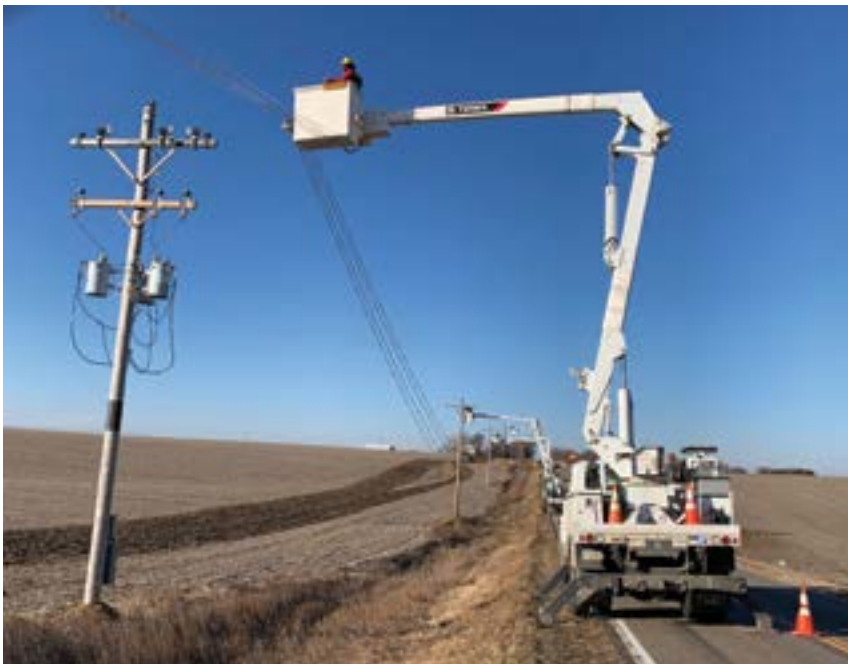
Crews stringing line on the Enola Road in December. This was a scheduled work plan project to help strengthen the system. ~Photo Credit: Patrick Hintz
