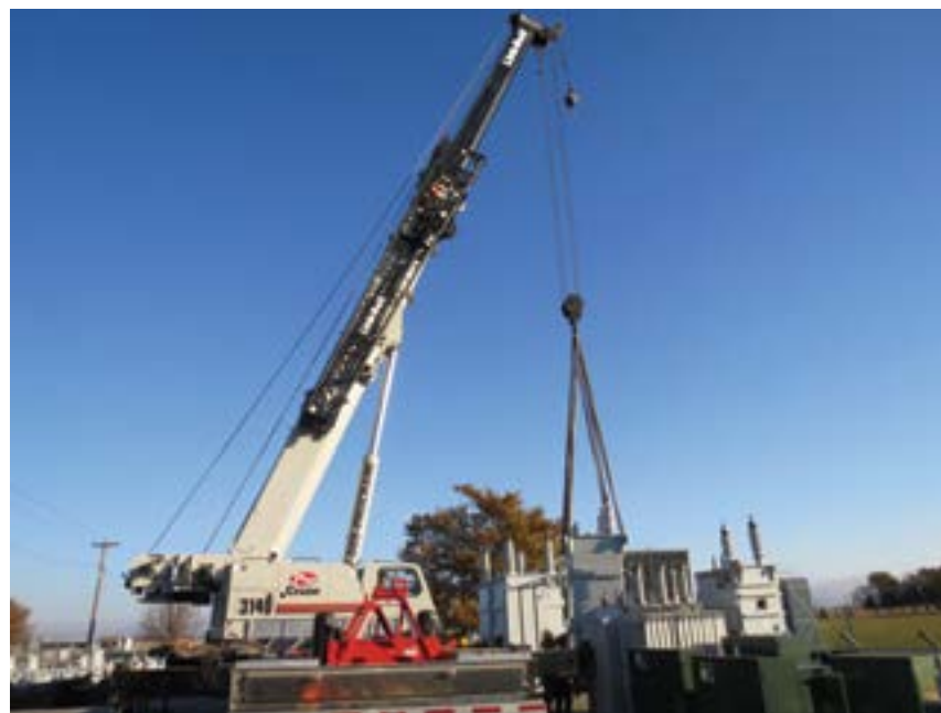
Pictured above: Crane unloading a substation transformer. It is part of ERPPD's plan for reliability.
