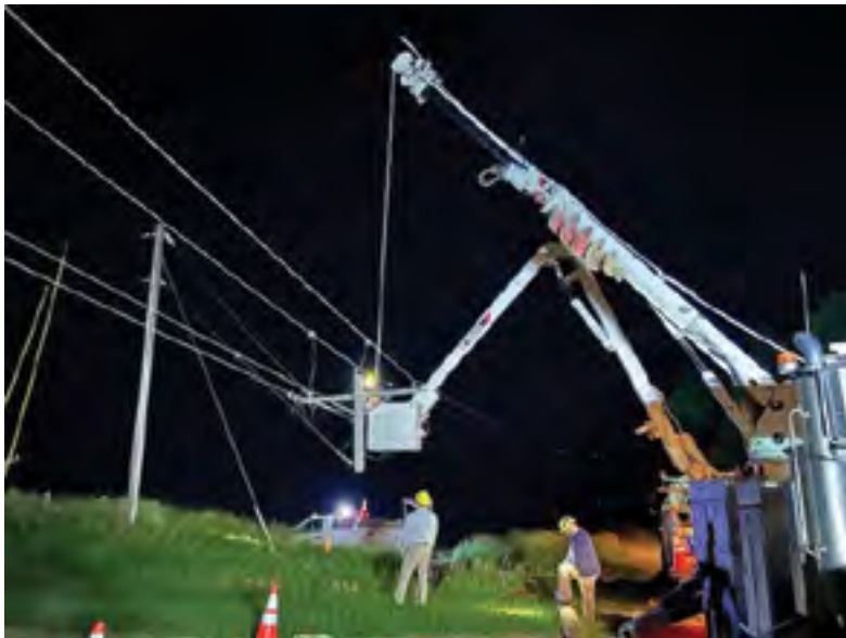
Crews working to repair line after a car accident in rural Pierce county.
