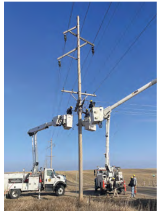
Crews work to install services and maintain ERPPD's electrical grid, efficiently. This helps with capacity, reliability and the cost-effectiveness of your electrical service.
