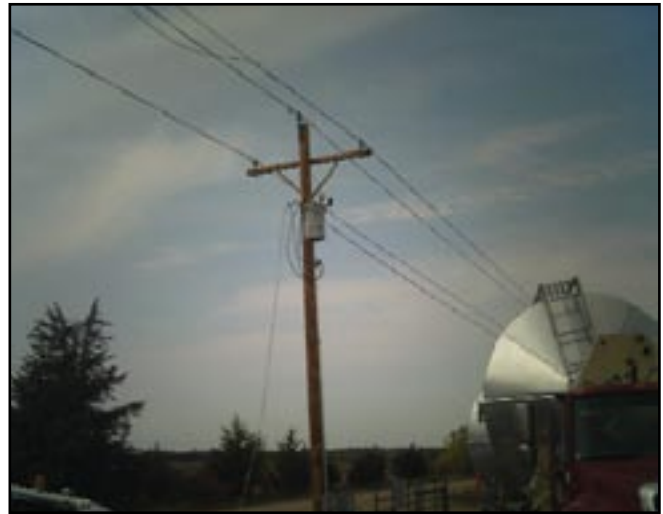
Photo shows neutral wire burned completely down and the phase wire burned nearly in two.
