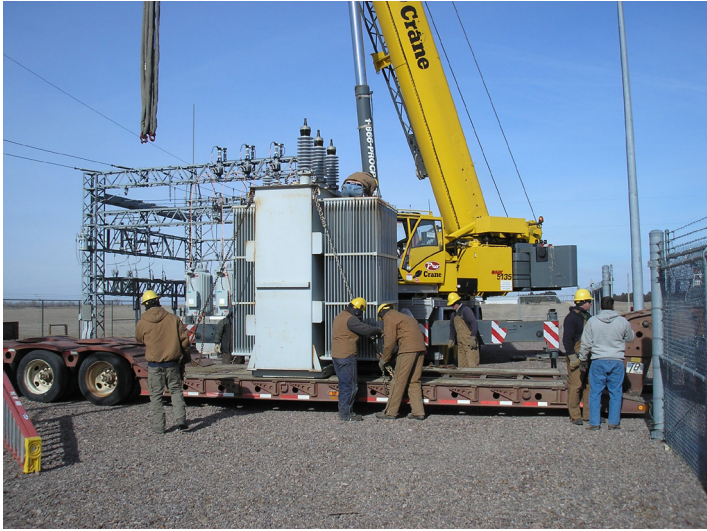
ERPPD crew members preparing a transformer to be lifted into position in Sub 19, five miles west of Elgin.
