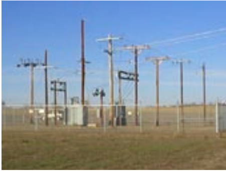
Temporary Miller Substation, built in 2004 and retired in 2012
