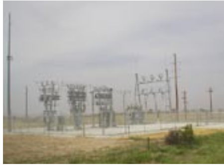
Permanent Miller Substation, built in 2012 and ready to serve the future needs of the area.
